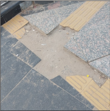
Prone to crack
