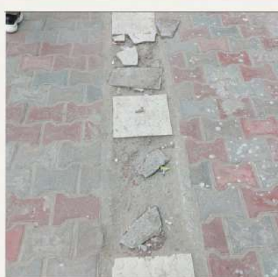
Installation takes a lot of time
