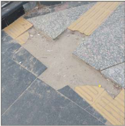
Prone to crack
